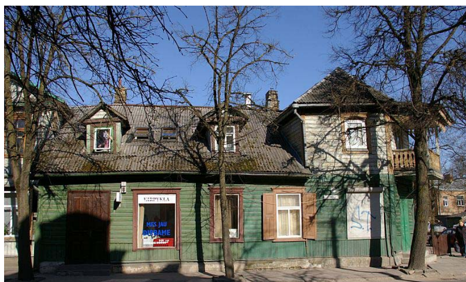
11 fig. Inappropriate restoration of windows. Vytauto 37/Pušų 9. Listed house.
